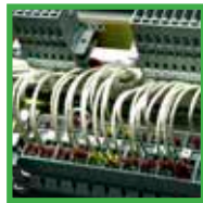
Electrical cabinets and substations
